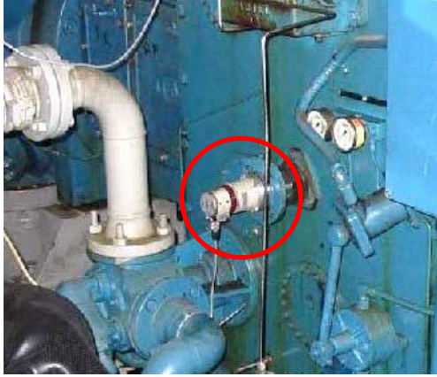
Figure 5 – HBM Torsiograph on Auxiliary End of Compressor
