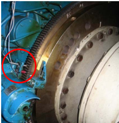
Figure 3 – Proximity Probe at the Engine Flywheel
