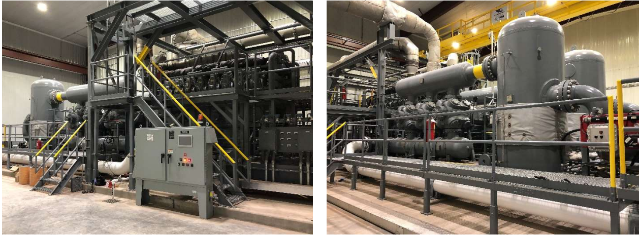
Figure 17. Engine Driven Compressor Unit
